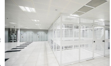
Equinix Stockholm IBX data center*
