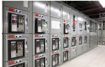
Equinix Stockholm IBX data center*
