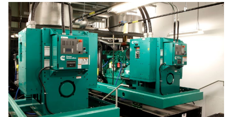
Representative Equinix IBX data center interior
