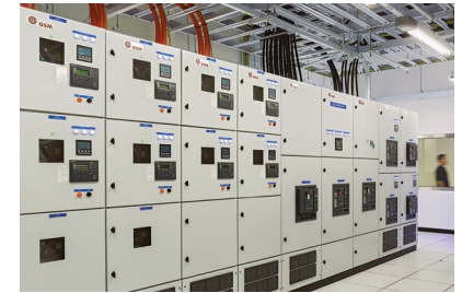
Representative IBX data center interior
