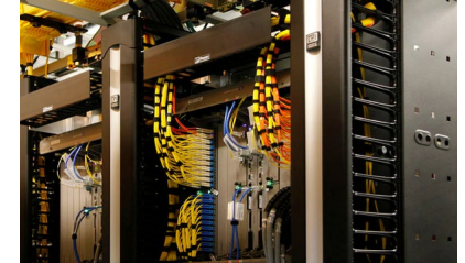
Representative IBX data center interior
