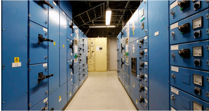
Equinix SK1 IBX data center interior
